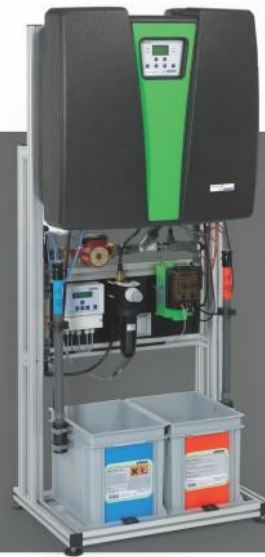
Drinking water disinfection
