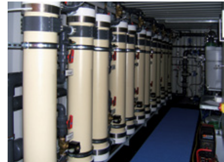
■ Filtration modules in a container-based system
